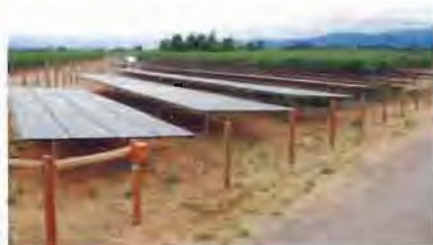
Sunlight Electric installed Honig Winery's 819 PV panels 1/4 mile from the winery buildings, on low-productivity land not in use for vineyards.
