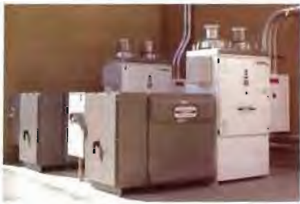
At 95% efficiency, Fetzer's Xantrex inverters and transformers convert DC current from PV panels to AC current for the utility grid.
