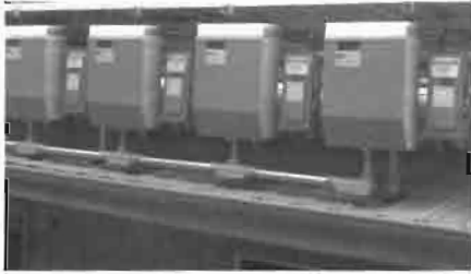
System inverters (brand is PVPowered, model PVP2800) mounted by REC Solar on back of solar panel racks at Raymond Burr Vineyards (Healdsburg, CA). Inverters convert DC to AC electricity and are the control units of the PV system. Photo courtesy Chris Bunas, SolarCraft.
