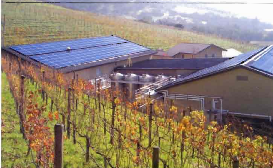
129 KW solar system at Shafer Vineyards, Napa, CA. Two arrays face east, two face west, and the ground mount (top right of photo) faces south for maximum exposure of panels. Photo courtesy Premier Power
