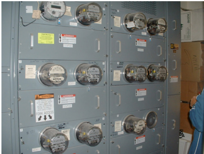
Figure 2: Customer's electrical closet: Before installation of solar
