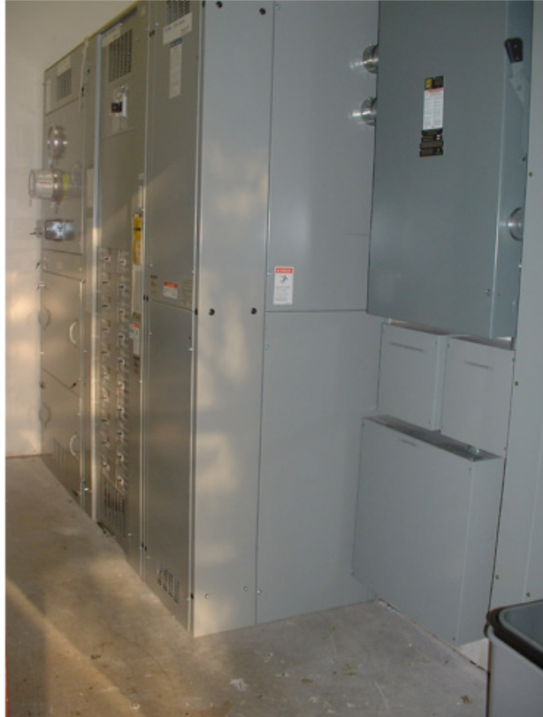
Figure 3: Customer's electrical closet: After installation of solar
